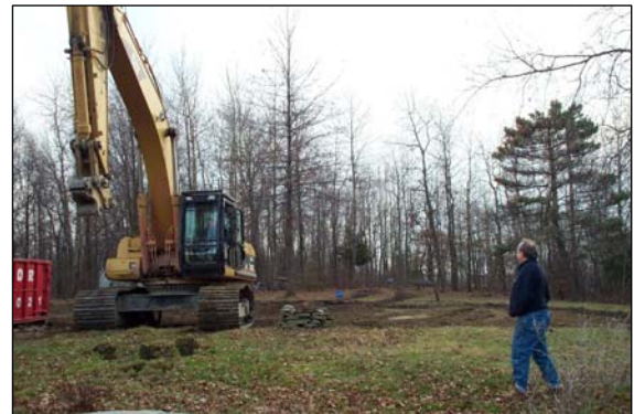
Top: Demolition of the burned out facility in progress. Bottom: The Rev. Jim Bridges watches as the demolition is completed.
